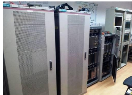
Linie BTS-BSC GSM/GPRS & NodeB-RNC 3G/UMTS– Siemens/NEC
